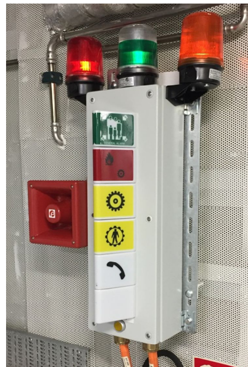
Photo 11. The four different standard emergency evacuation signals. They have not been altered with the implementation of batteries.
