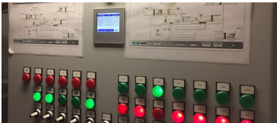
Photo 7. The ventilation system.
