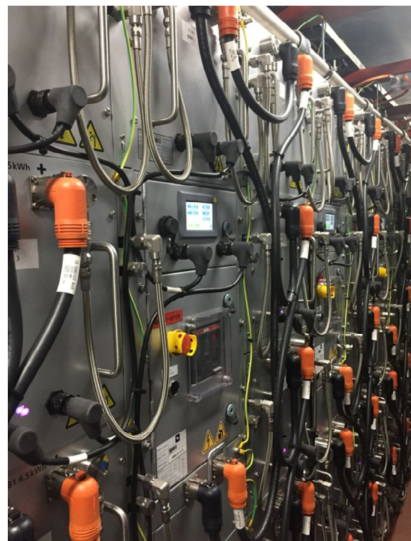
Photo 3. Batteries on "Electric"
